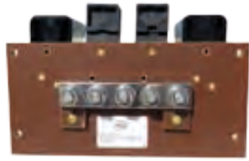
NZI 60A 4 Way Domestic Panel – Back View
